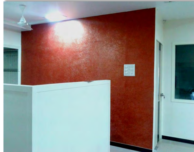
Wall Paneling - (V-Board)
